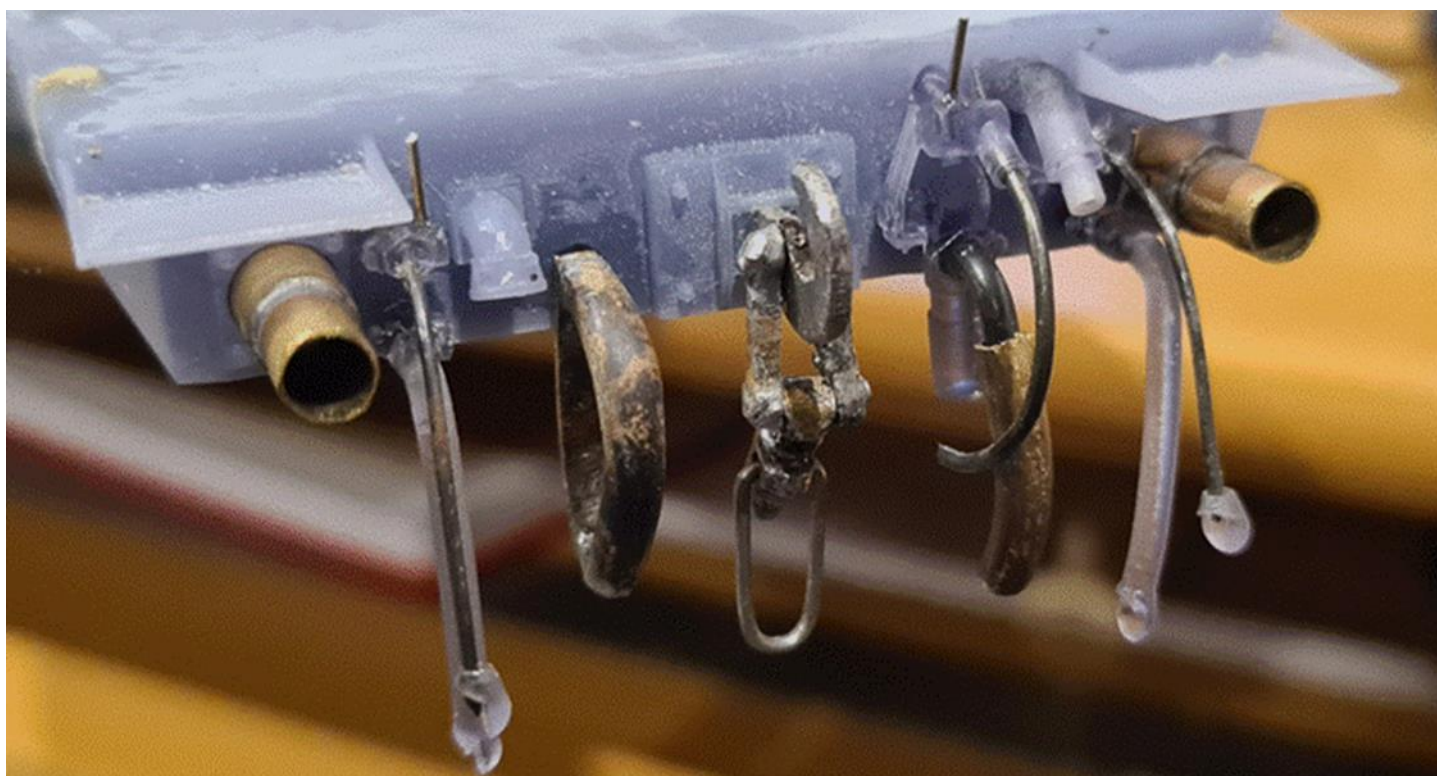
The array of hoses and cables fitted to one of the buffer beams. N.B. the buffers were removed to allow more access for fitting.
