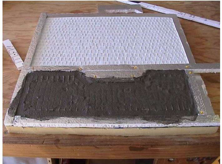
Mold with lower half filled. Note piece inserted at top to provide cut out to fit a dormer roof, and lines made by inserting the hardware cloth
