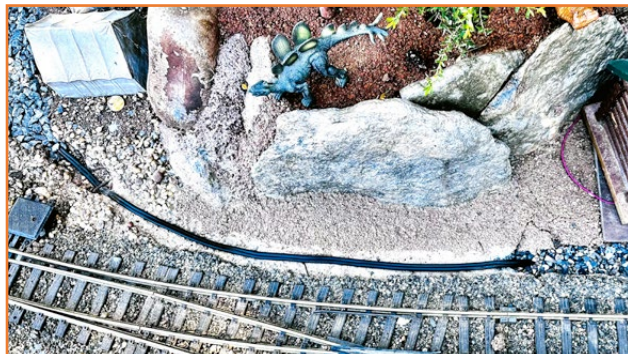
New lighting circuit being laid under the watchful eye of a random dinosaur..
