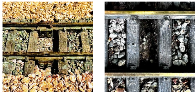
Water can collect if ballast is missing, causing a track short.
