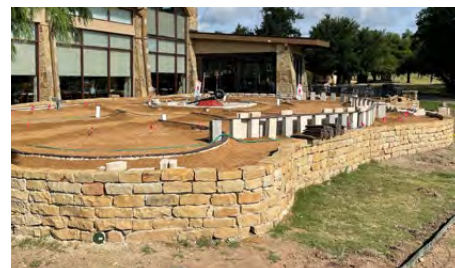
Upper track support blocks.
