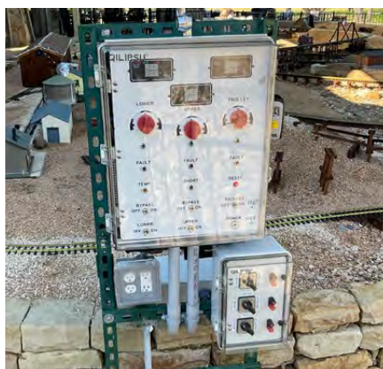
Main control panel and back-up sub-panel.
