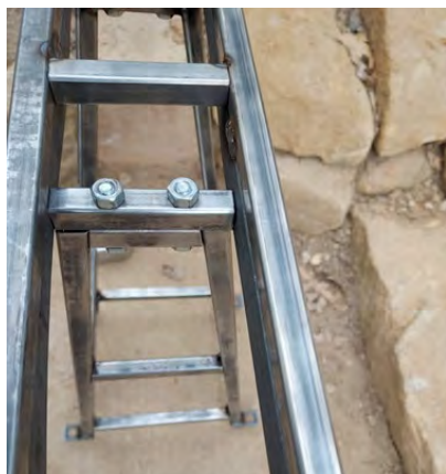
Photo 11 Lining up the A-frame tower to the deck to weld crossmember to rail.
