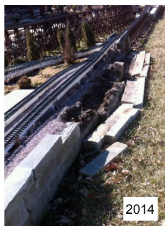
Frost Heave Damage
